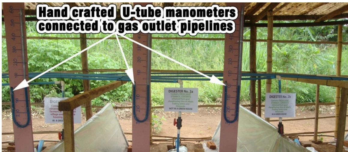
Figure 10: U-tube manometers connected to gas outlet pipe line
